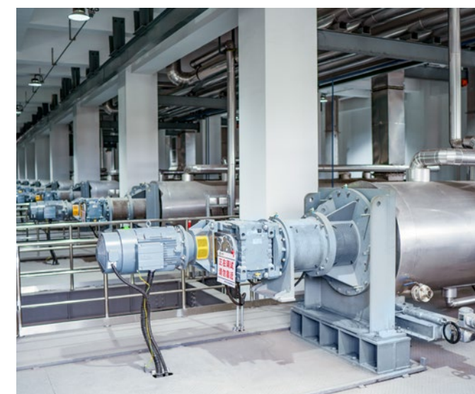
Zhuyuan Sludge Treatment Plant of Shanghai Chengtou Sewage Treatment Co., Ltd
